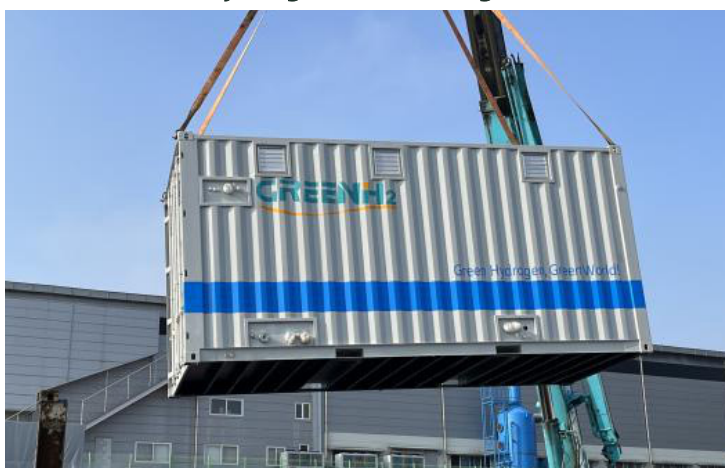
Hydrogen Generating Plant
